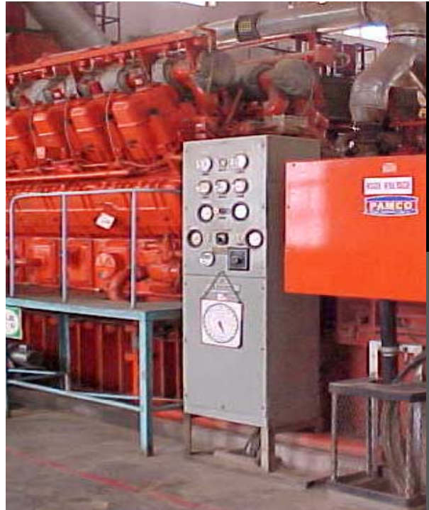
WAUKESHA 12V-AT25 GL Gas Engine Lubricated with Mobil Pegasus 705
