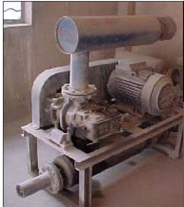
Roots Blower in Zhujiang Cement Plant
